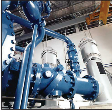
Tilted Disc® Check Valve with Well Service Air Valve on Vertical Turbine Pump.
