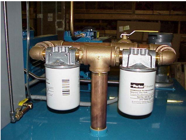
FIGURE 9. Typical Return Filters
