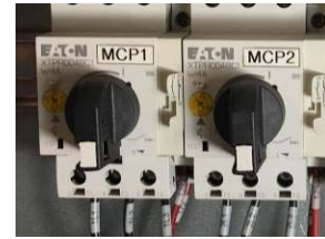
Figure 11. Motor Starters. Shown in Normal (untripped) Position
