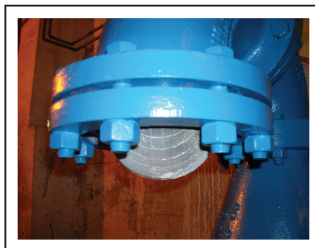
VentSafe® Security Cage Installed on Vent Pipe
