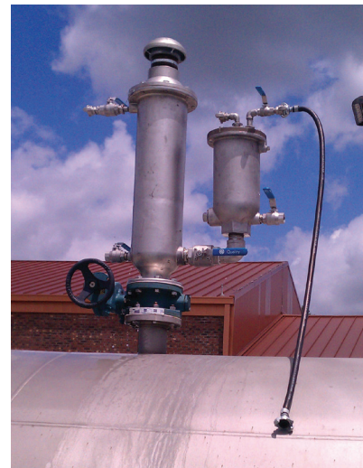
Lithia Water Treatment Plant Tampa, FL
