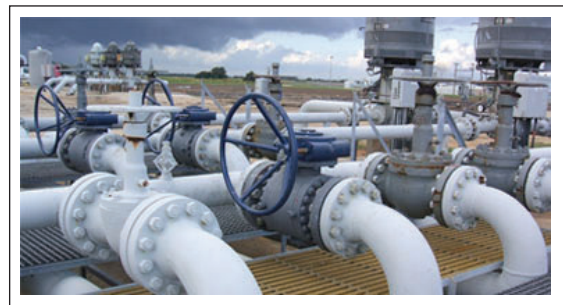
Salt Dome Brine & Gas Pumping Station
