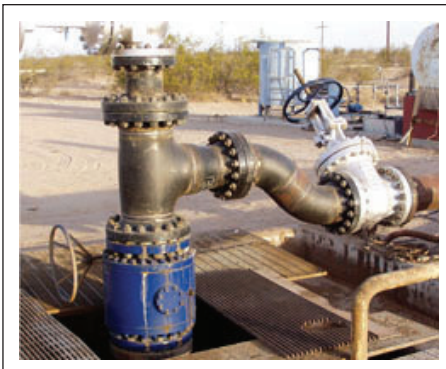
Master Valve Geothermal Brine
