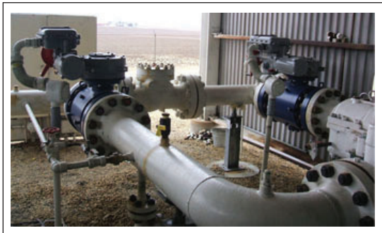
Crude Oil Pumping Station Pig Launcher/Receiver
